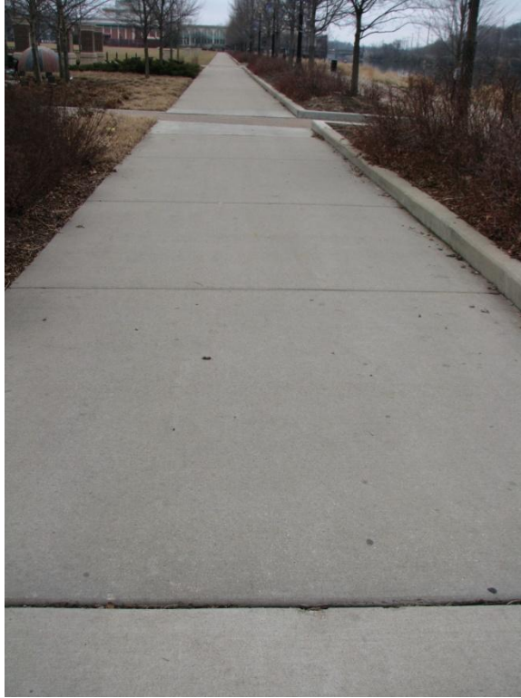
Figure D.46. Typical PCC pavement section with some joint spalling.
