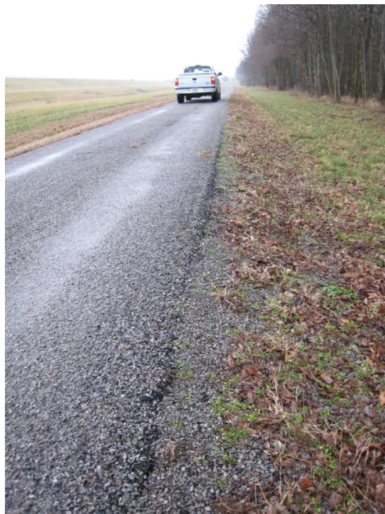
Figure D.28. Rutting and breakdown at the edge of the bituminous surface.
