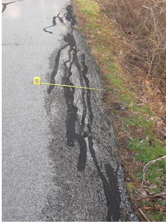
Figure D.32. Area of edge cracking and fall-off.
