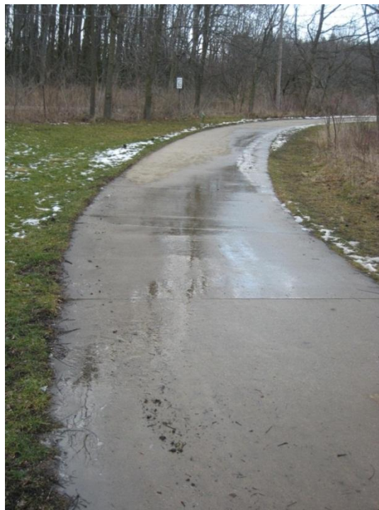
Figure D.4. Lack of trail drainage.
