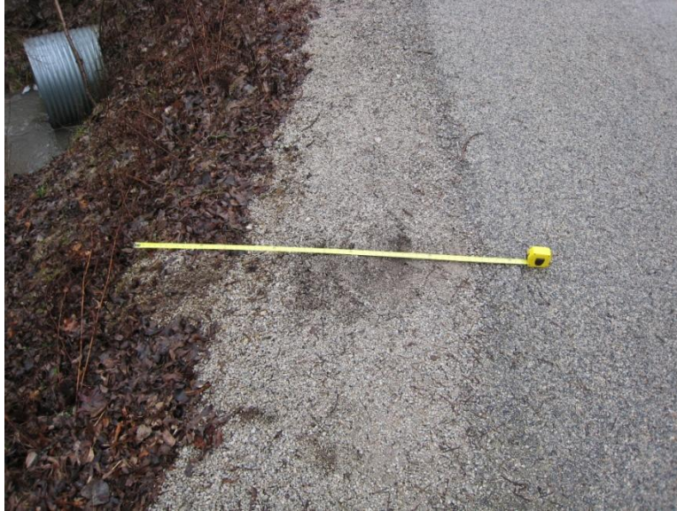
Figure D.10. Aggregate base extended beyond the edge of the surface treatment.
