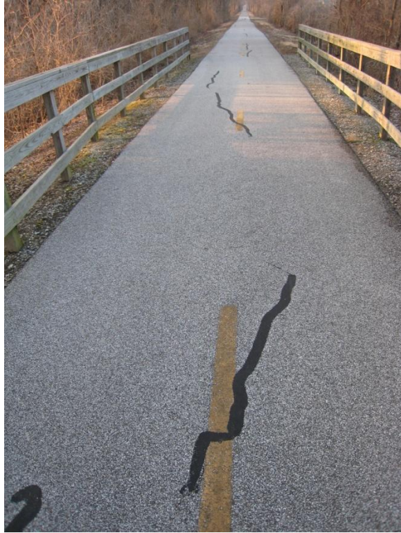
Figure D.39. Low-severity longitudinal cracking.
