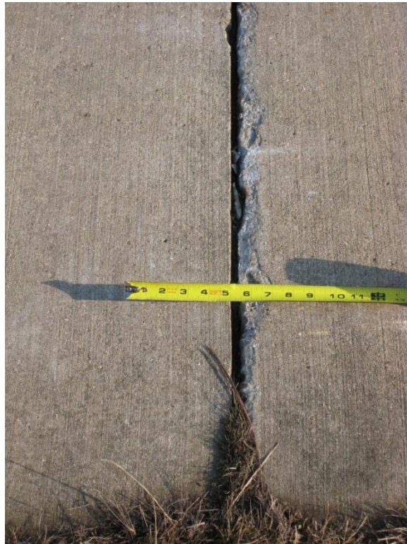
Figure D.2. Joint faulting leading to further deterioration.
