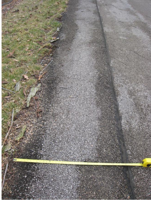
Figure D.34. Patch correcting edge cracking.
