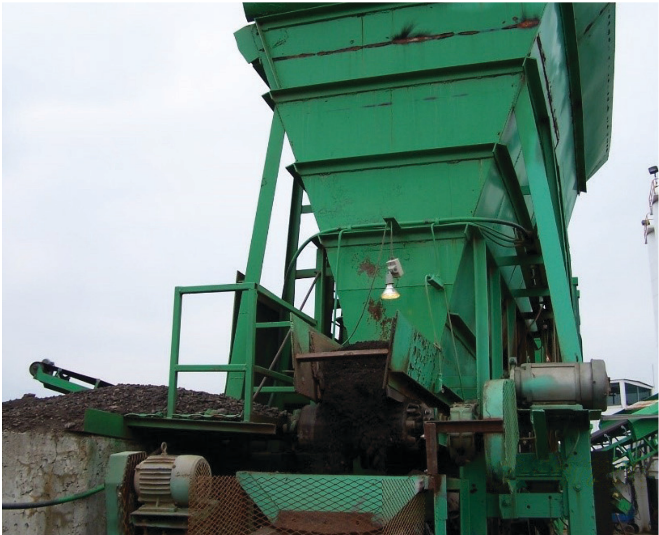
Figure 4-1. Steep-sided RAP cold feed bin.
