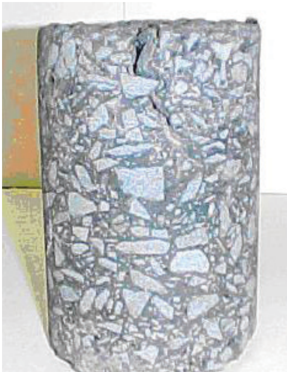
Figure 1-2. Roadway cores showing distressed layers: top-down cracking on top; stripping damage on the bottom.
