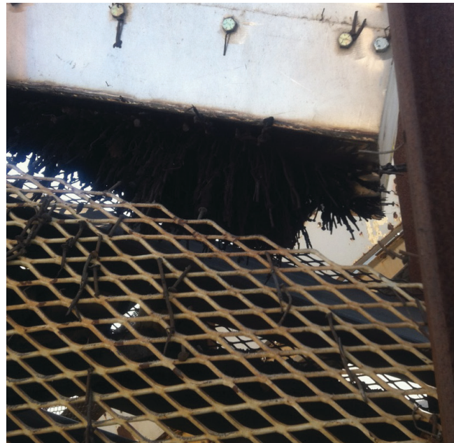
Figure 5-3. Magnet used to remove nails from RAS feed to the asphalt plant.
