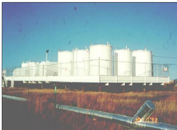
Figure 3-1: Fencing around oil storage area.
