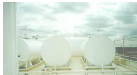
Figure 7-3: Shop-built containers elevated on saddles.
