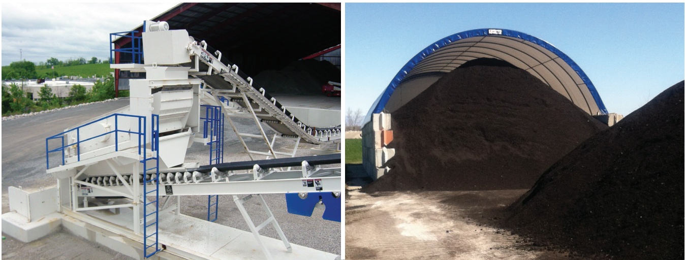
Figure 12. Two examples of covered processed RAS. At left, the RAS is stored on a paved surface with the RAS feed system in the foreground.
